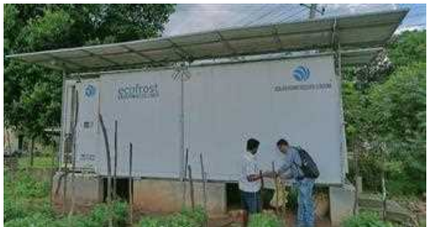
Outer view of a 5MT refrigeration unit at Anekal
